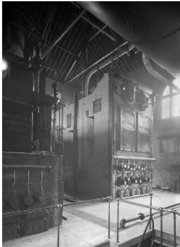
Figure 31. Interior of the Boiler House, December 8, 1915, looking northeast, showing Boiler No. 3 (right). The inscription on the cast iron doors of the boilers reads "Edgemoor Iron Co. — Edge Moor — Delaware" (Historic Pittsburgh).
