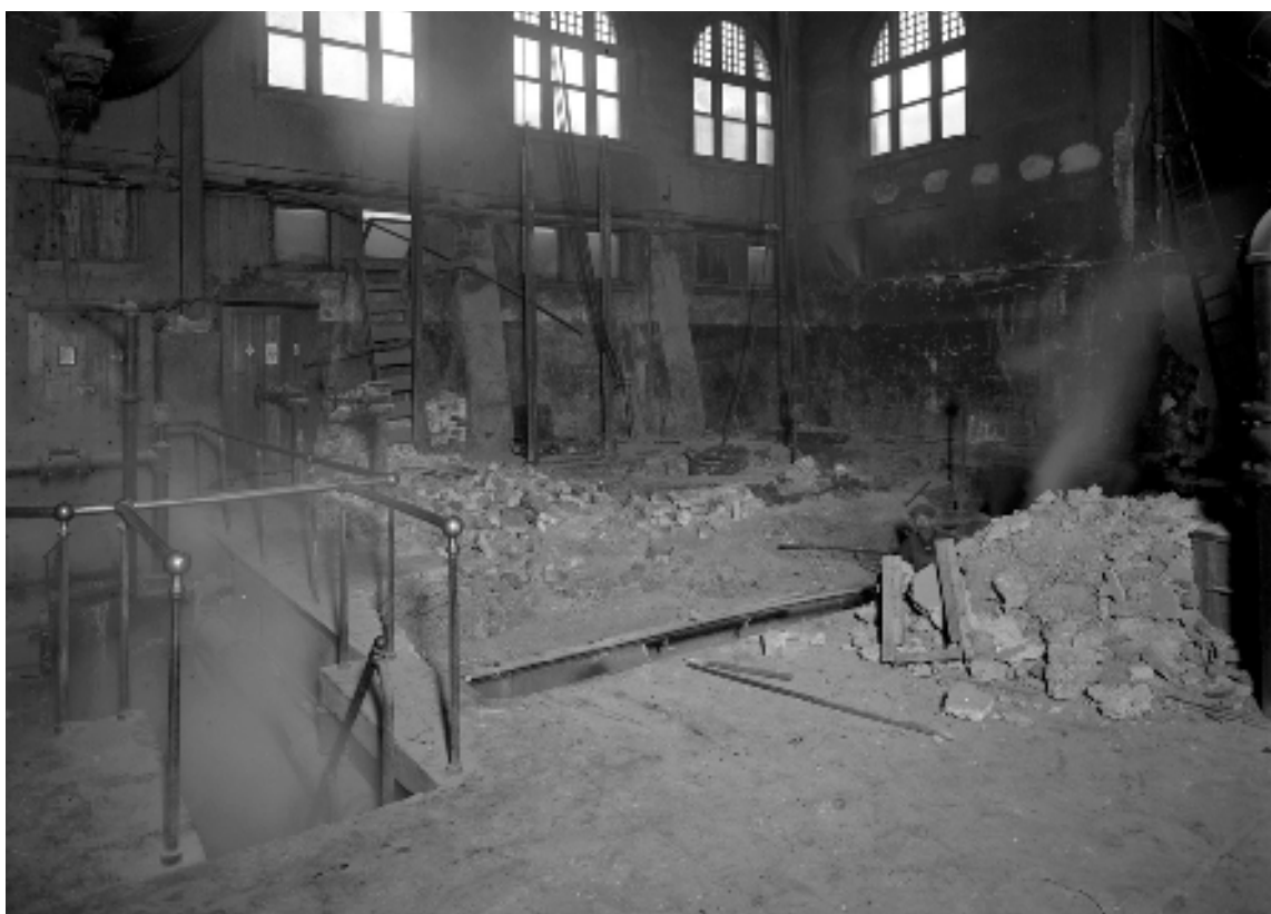
Figure 32. Interior of the Boiler House, January 8, 1919, looking northwest, showing demolition in preparation for new brick boiler foundations (Historic Pittsburgh).
