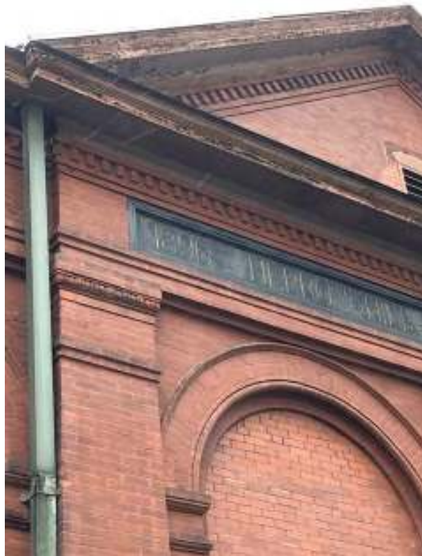
Figure 13. Detail of the front facade of the Pumping Station Building, showing a pilaster with Tuscan capital and egg-and-dart molding; the frieze containing the name and date of the building; and the triangular pediment above with its raking cornice of brick dentils.
