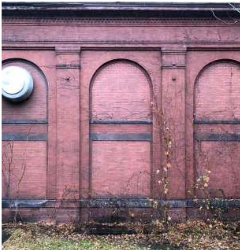
Figure 11. West wall of the Pump House, showing typical red brick walls and Classically-derived pilasters with Tuscan capitals supporting a simple entablature above.
