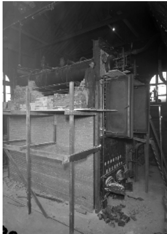
Figure 35. The same boiler on February 18, 1919, showing erection of its new brick foundation in progress (Historic Pittsburgh).
