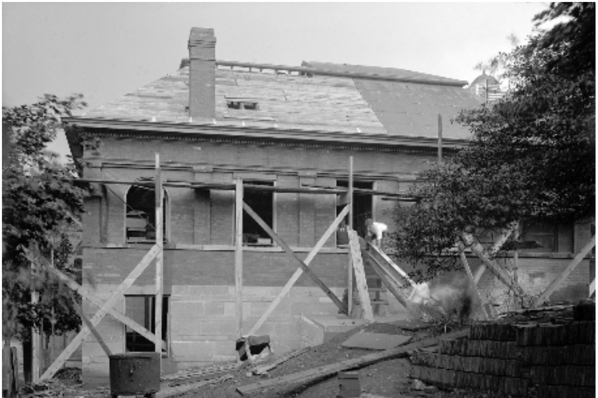
Figure 45. North facade of the Laboratory Building in 1909, looking south, showing the new roof being constructed (Historic Pittsburgh).
