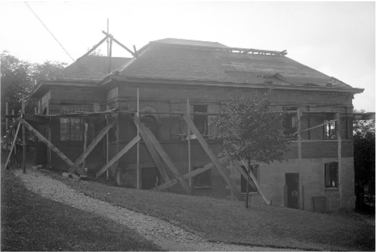
Figure 44. South facade of the Laboratory Building in 1909, looking north, showing the new roof being constructed after the top floor of the building was removed (Historic Pittsburgh).
