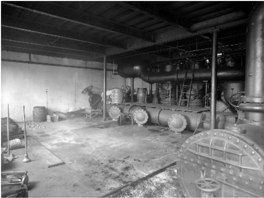
Figure 28. Ground floor of the Pump House, October 17, 1919, showing the water distribution pipes (Historic Pittsburgh).
