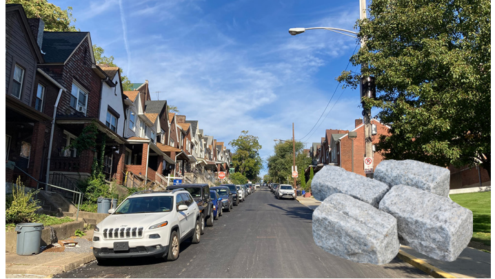
PWSA has paved Chesterfield Road for now, but will replace the Belgian blocks in spring.
