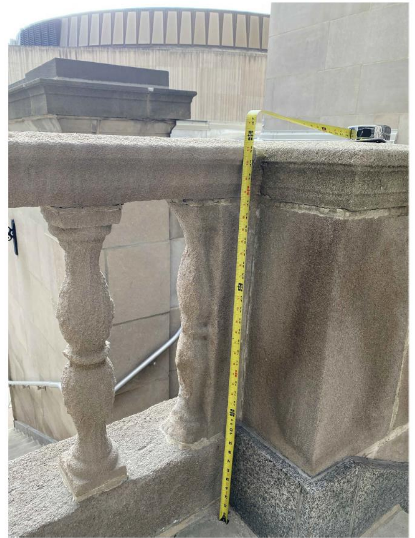
3 EXISTING DETERIORATED LIMESTONE BALUSTRADES
